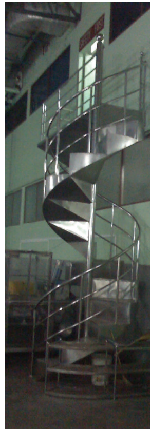
Stainless steel Spiral ladder for emergency exit.
